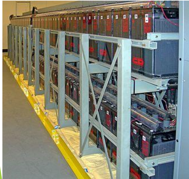
Electrical power Installation
