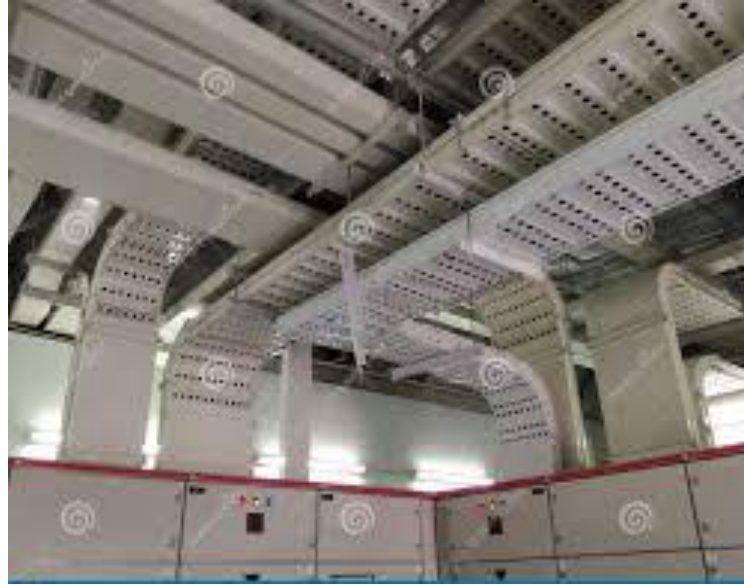
Low-voltage cable routing Services
